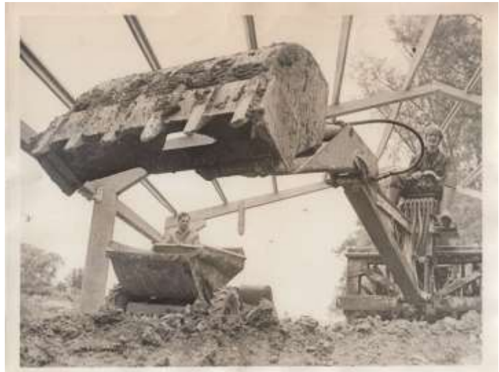
Digging Ridgemedede School swimming pool 1975 John Watts (headmaster) in dumper truck, Mark Weller (parent) in the digger. John Bosworth (BW01102416)
